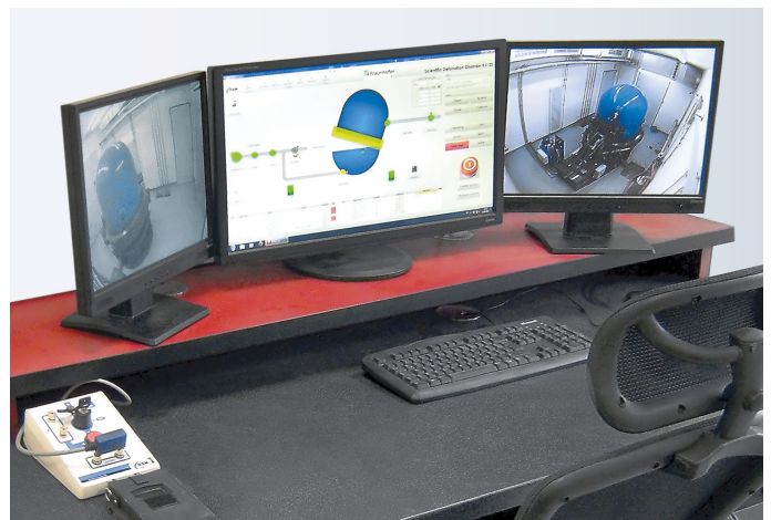
Control panel of the detonation chamber
